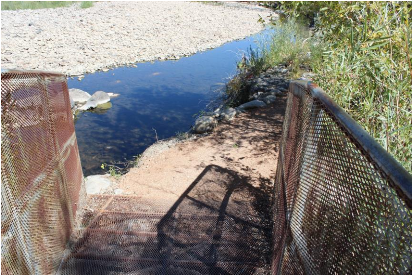
Photo 2: Severely eroded bank looking east from the Minnesota Creek Bridge is a safety and ADA compliance risk, and a threat to bridge stability.
